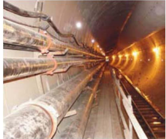
14" and 16" R-88 couplings used at the Eastside Combined Sewer Overflow Tunnel Boring Project – Portland, Oregon, USA.
